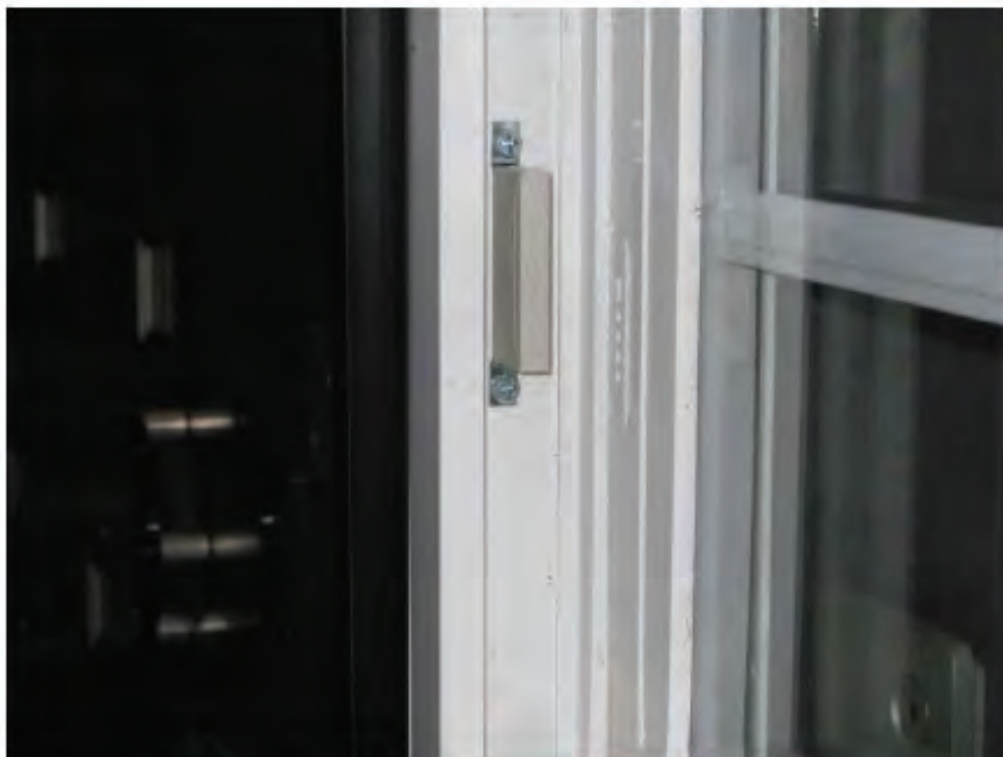
Photo No. 2 View of Window Opening Limiting Device No. 1
